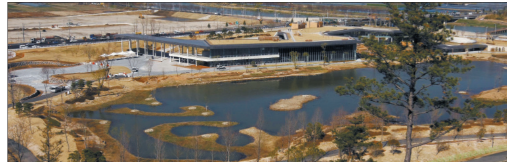
(From top) A garden in the Netherlands is one of those featured at the Suncheon Bay Garden Expo; various landscaping and installation works; the Suncheon Bay International Wetland Center. The six-month garden expo, the first of its kind in Korea, kicks off Saturday and includes gardens by several international designers. Provided by the organizers
